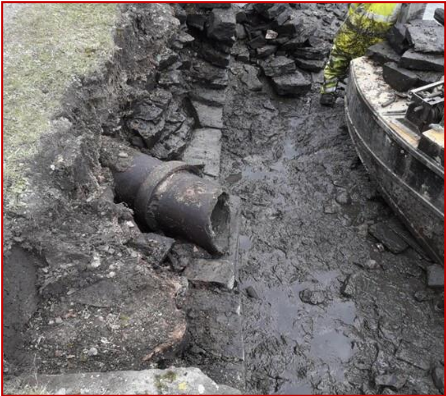
The problem uncovered!
